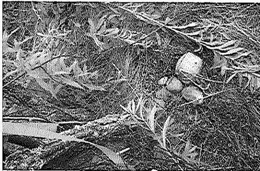
Mound of Rocks at rotted off end fence post near South right-of-way
